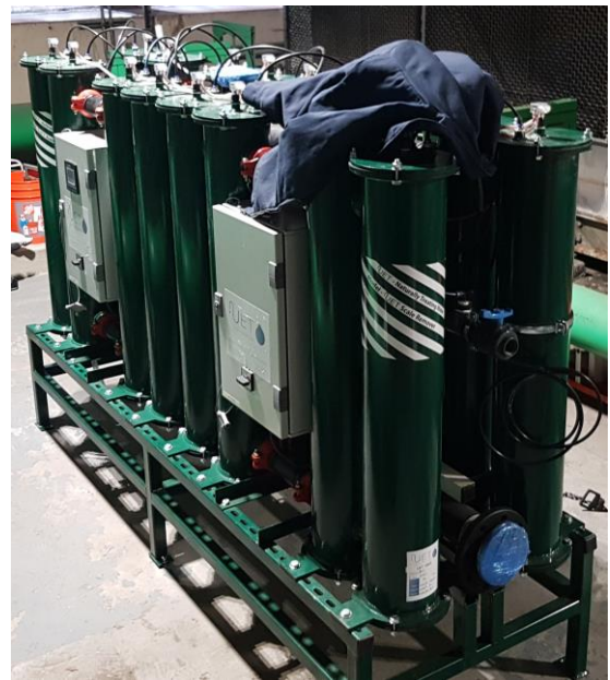
The UET unit treating cooling towers on site
